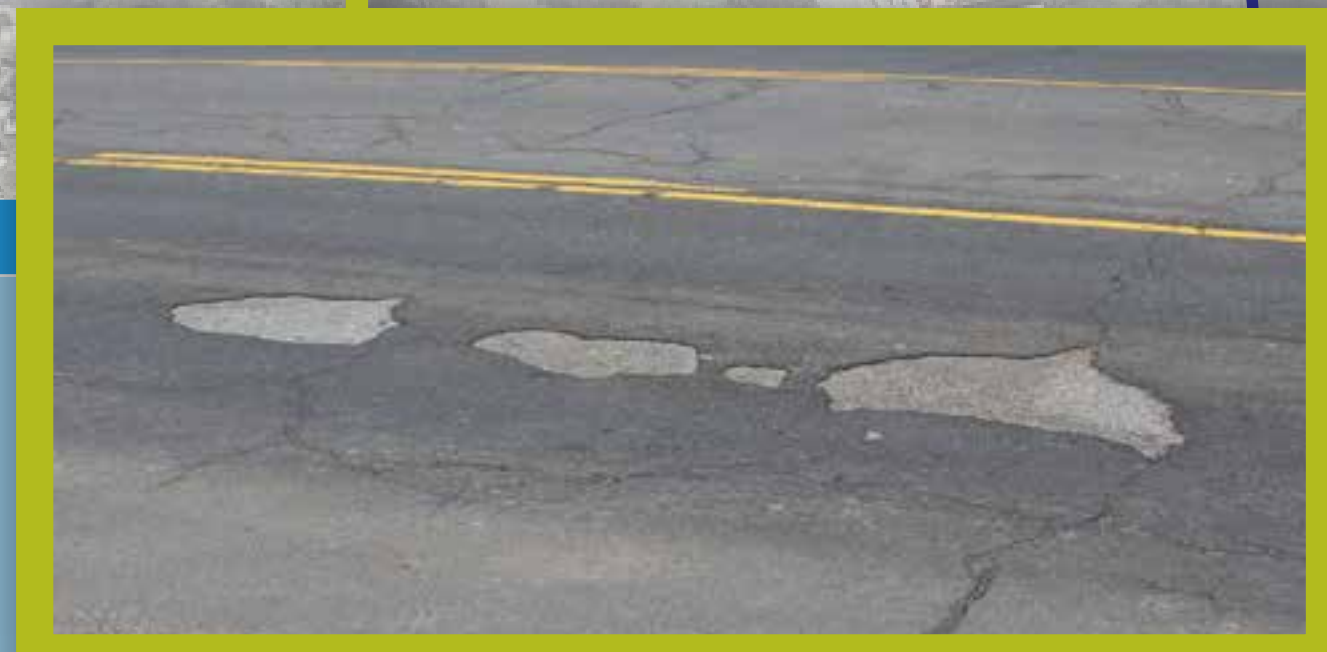
Pavement along the corridor shows its age. The project will include regrading and repaving along the corridor.
